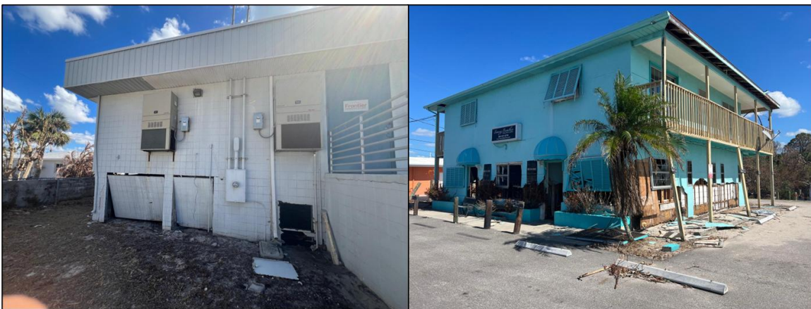
Figure 8: Low-rise commercial buildings, near the coastline, suffered damage to exterior walls and windows due to storm surge in Manasota Key.
