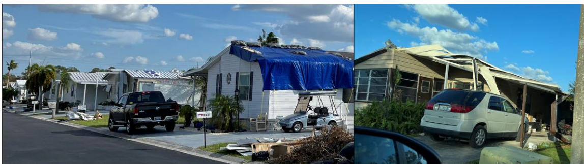
Figure 9: Widespread roof damages for mobile/manufactured homes in Hillsborough County.
