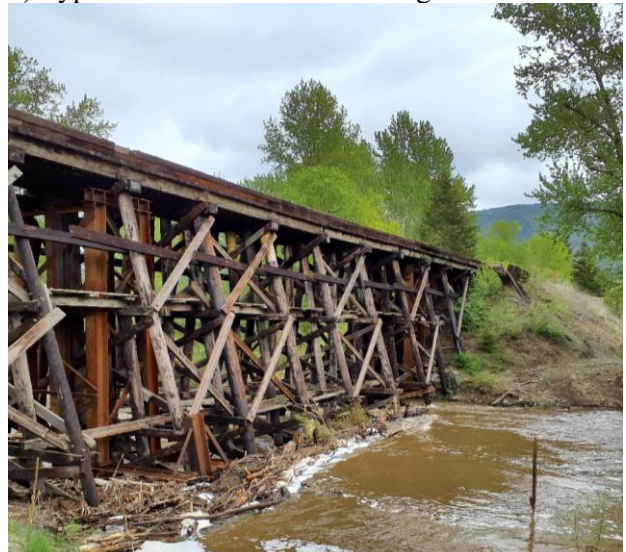
d) Wood trestle bridge accumulating debris.
