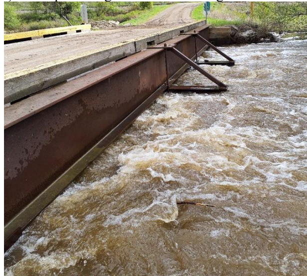
c) Low clearance farm bridge experiencing pressurized flow.
